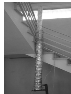
Fig. 9. A picture of the vertical insulated pipe.
